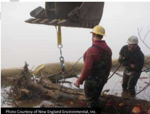
Photo Courtesy of New England Environmental, Inc. Testing the stability of the large woody debris structure
