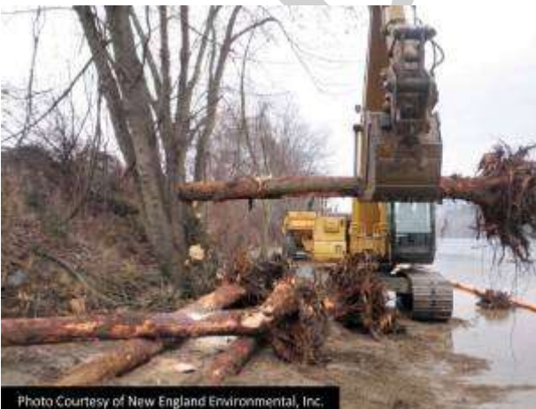
Photo Courtesy of New England Environmental, Inc. Construction of the large woody debris structure
